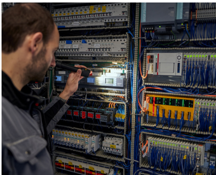
Reverion's electrical equipment relies on the expertise of, among others, HELUKABEL.
