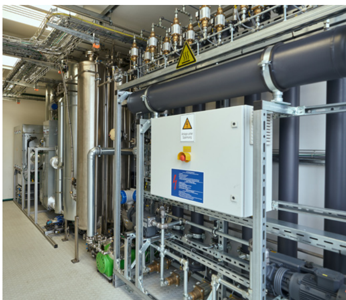
The system can be switched to an electrolysis mode, which allows electrical energy to be used to produce hydrogen and methane.
